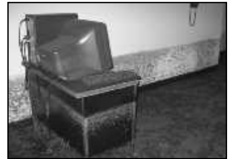
The most severe water damage to USM's Gulf Coast Library was in the computer lab. This picture shows the high-water line. The dark spots on the wall are mold. Photo by Barton Spencer
