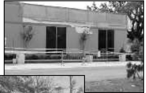
Damage to the roof of the Bay St. Louis Public Library. Photo by Gloria J. Washington
