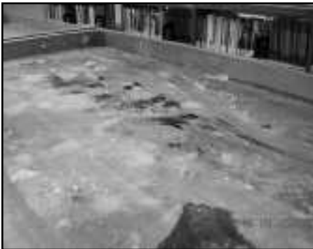
Water damage and humidity caused mold to grow in the stacks of the MGCCC libraries. Photo by Pamela Ladner
