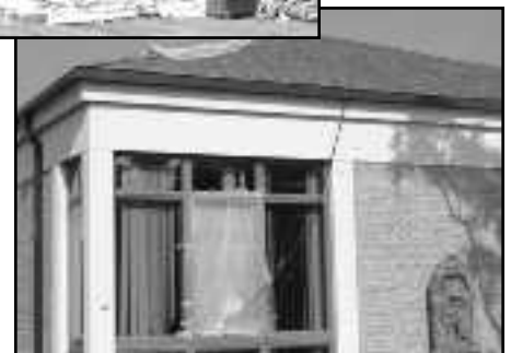
Roof and window damage to the Kiln Public Library. Photo by Gloria J. Washington
