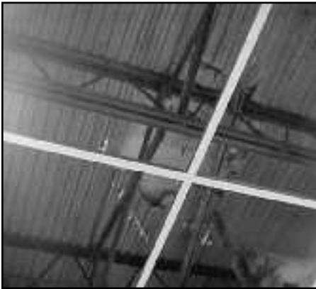
Katrina cause structural damage at the Jackson County MGCCC Library. Photo by Pamela Ladner
