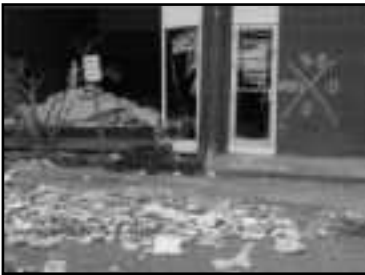
Damage to the side Long Beach Public Library; the red marks mean the building had been checked for survivors. Photo by Gloria J. Washington
