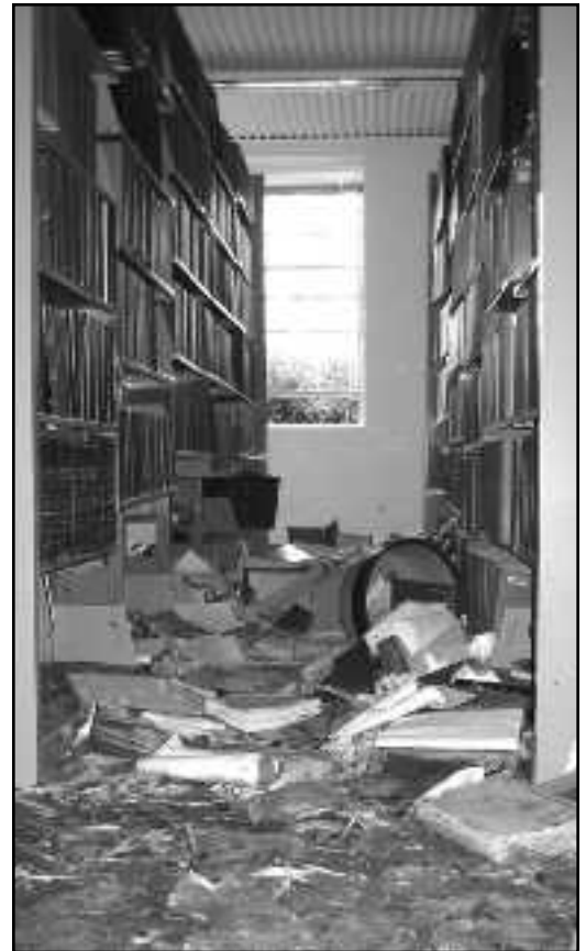
The floor of the library was covered with a layer of mud, sand, sewage, and books. Photo by Pat Yuen.
